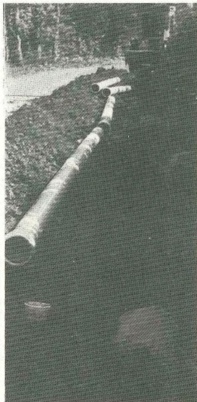
Randy Stark and Vance Hubbard lay P.V.C. pipe for the Corbett Water District.
