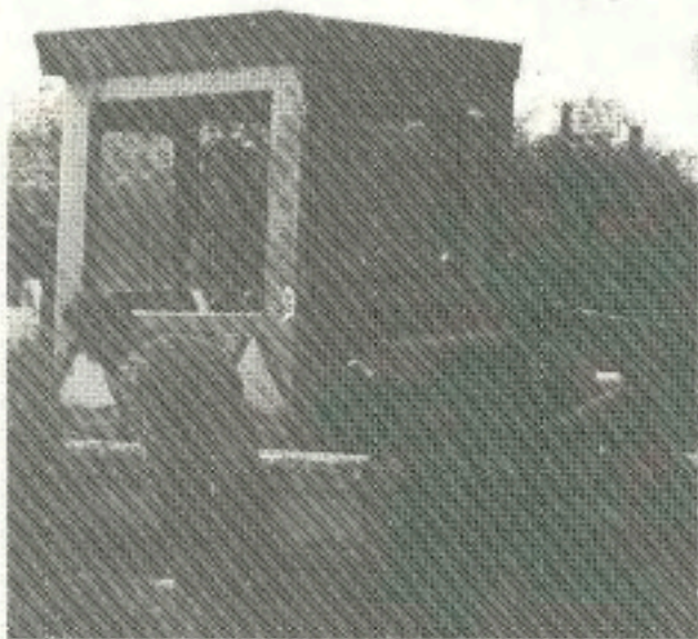
Dennis Granberg, who left the Water District in August, 1980, works with a backhoe to dig a ditch.
